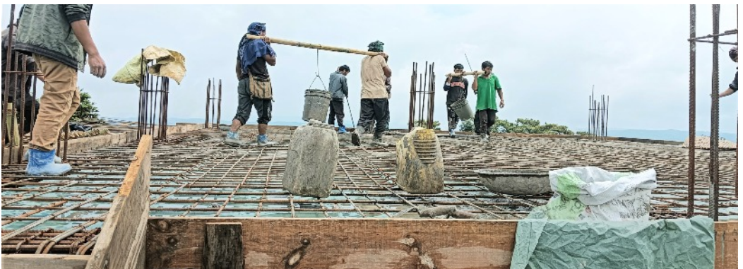
Work is now underway to restore the living Memorial to Margaret Barr
